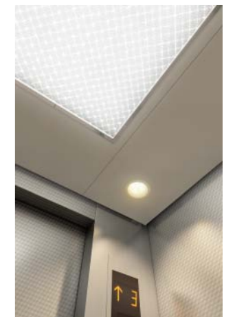
Ceiling: Painted steel sheet (Y033) with an acrylic lighting cover Lighting: Central lighting and downlights (LEDs)
